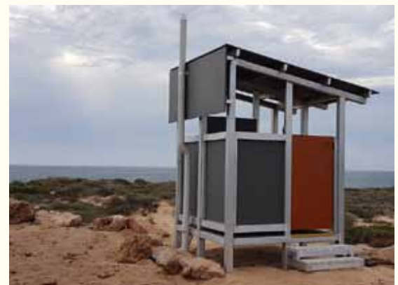
Left - Unloading a prefabricated toilet for transport across the island. Above - Loo with a view at Urchin Point.
